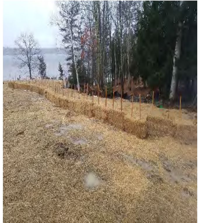
Fig 2: BMPs on slope at Getchell property/west side of the Bay, around area where previous erosion was observed. Viewing east. (02-27-20).
