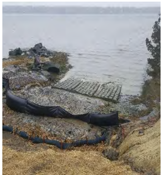
Fig 4: BMPs installed at toe of slope at Getchell property/west side of the Bay. Viewing east. (02-27-20).
