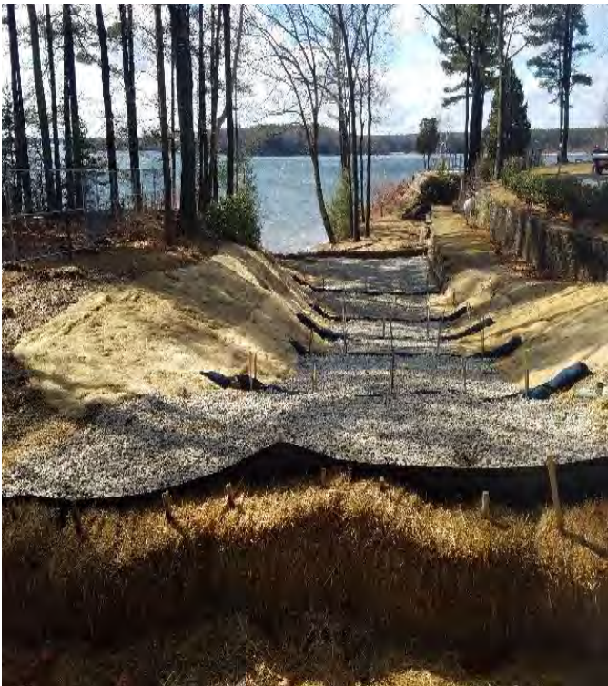
Fig 11: BMPs on slope to vault at Gundalow landing/east side of the Bay. Viewing west. (02-27-20).
