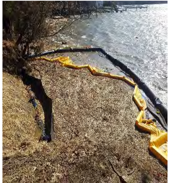
Fig 12: BMPs at toe of slope and turbidity barrier in intertidal zone at Gundalow landing/east side of the Bay. Viewing south. (02-27-20).
