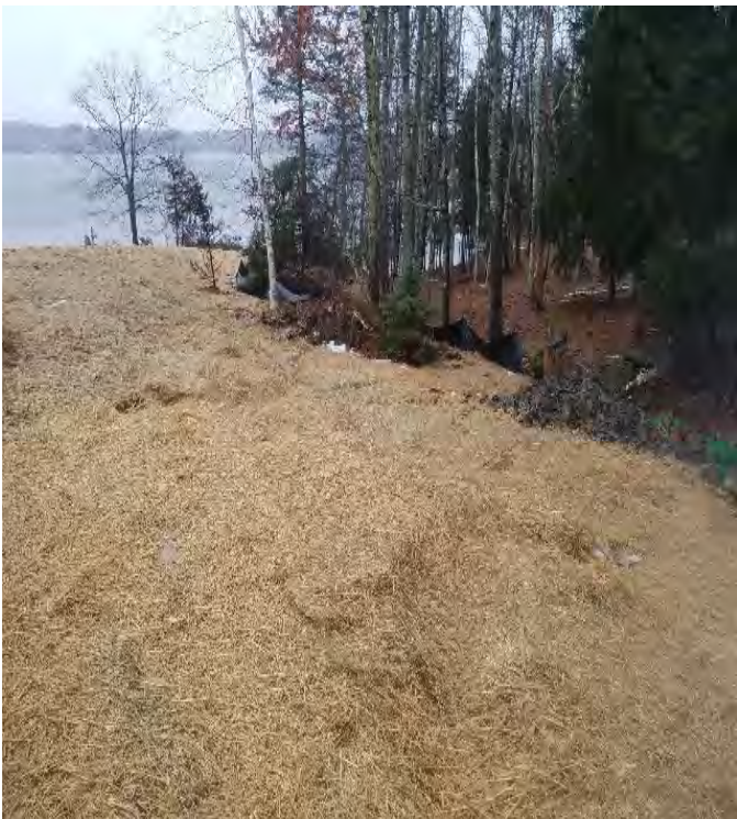
Fig 3: Erosion blanket preventing any further erosion at Getchell property/west side of the Bay. Viewing east. (02-27-20).
