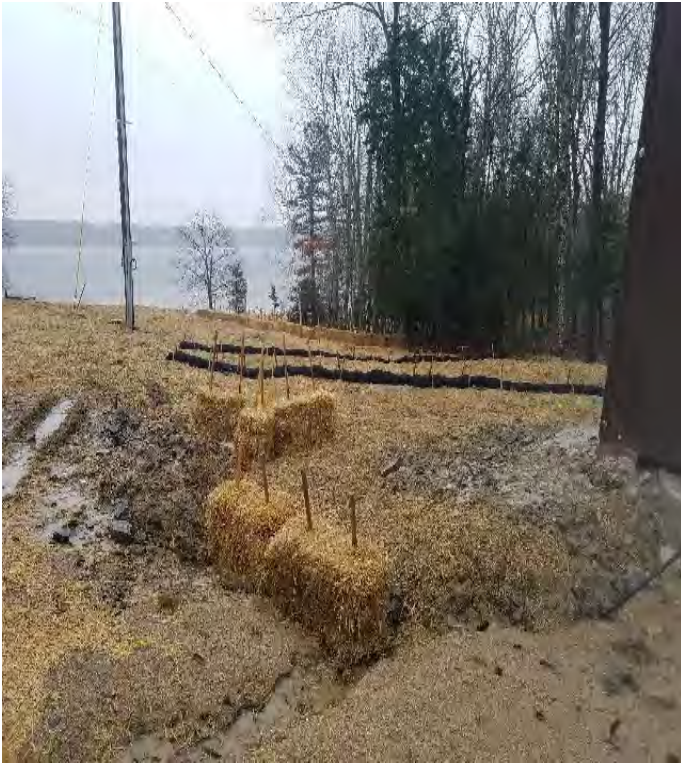
Fig 1: BMPs installed on slope at Getchell property/west side of the bay. Viewing east. (02-27-20).
